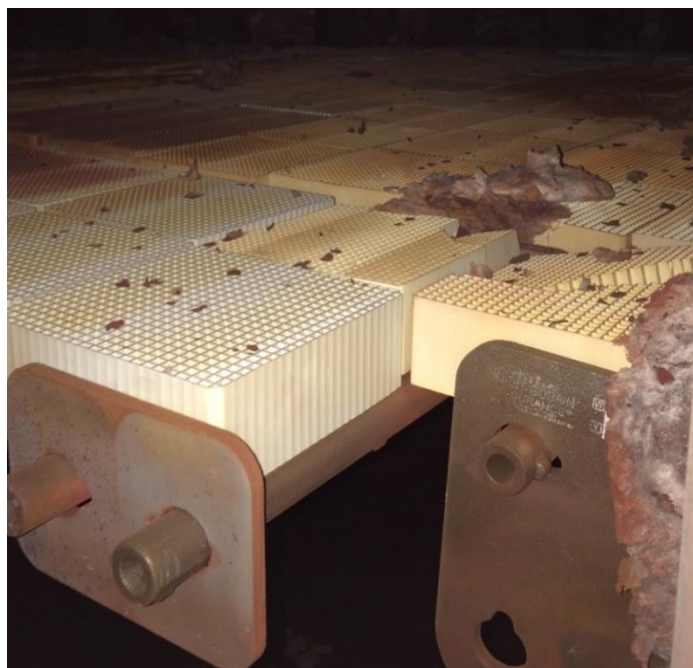
Figure 2: DUPLEX tile in process heater with minor damage to tile
