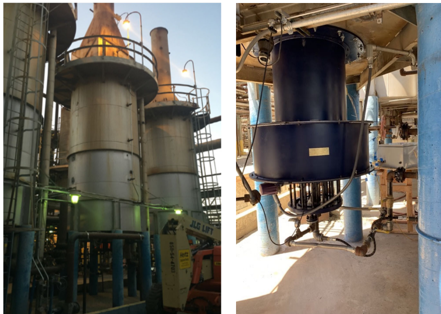
Figure 3: Refinery Process Heater (left) and ClearSign Plug & Play Burner (right).
