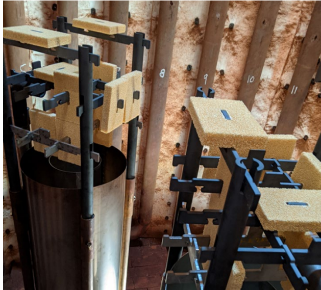
Figure 1 – Installed ClearSign Core Process Burners
