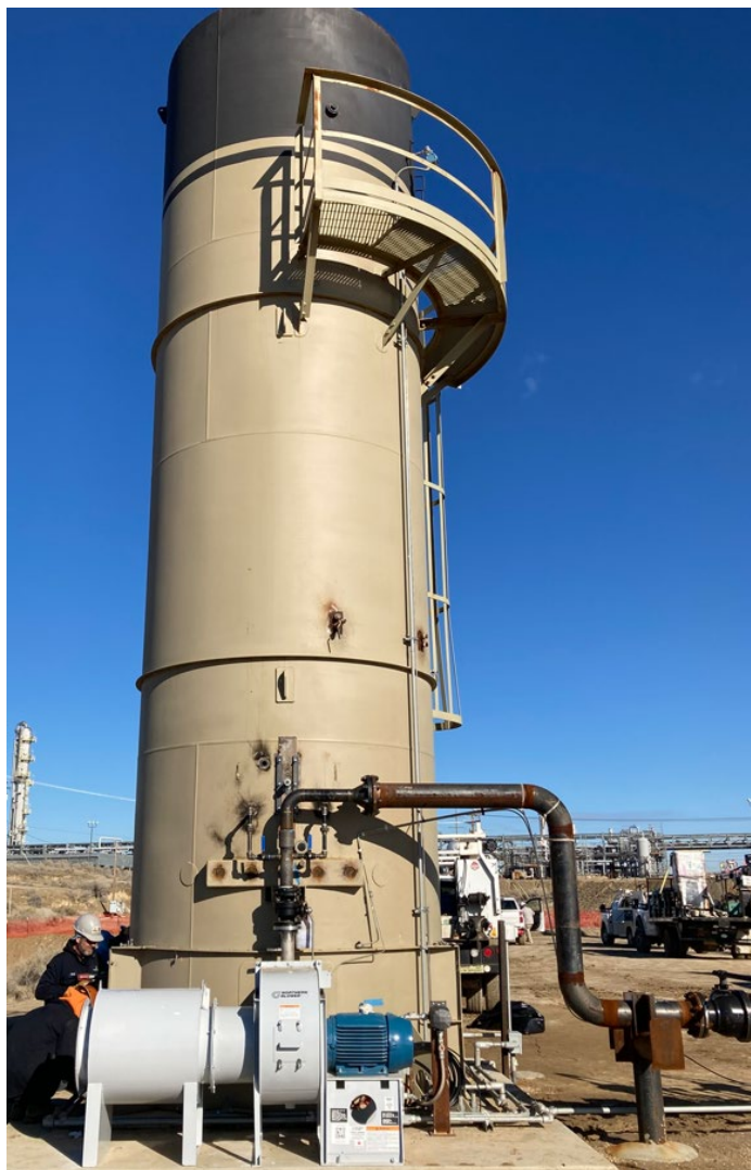
Figure 7 – Burner Installed in the Enclosed Flare Stack
